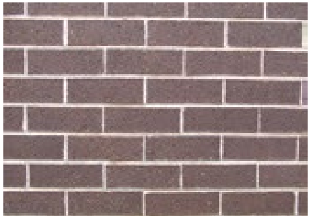
Figure 59 Damage caused by incorrect high pressure water jet cleaning
