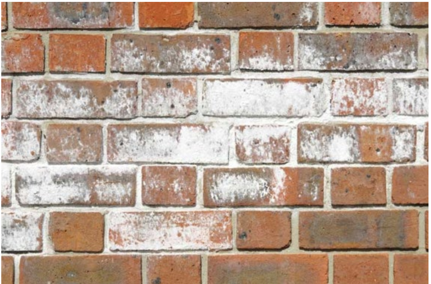
Figure 06 Effects of Efflorescence
