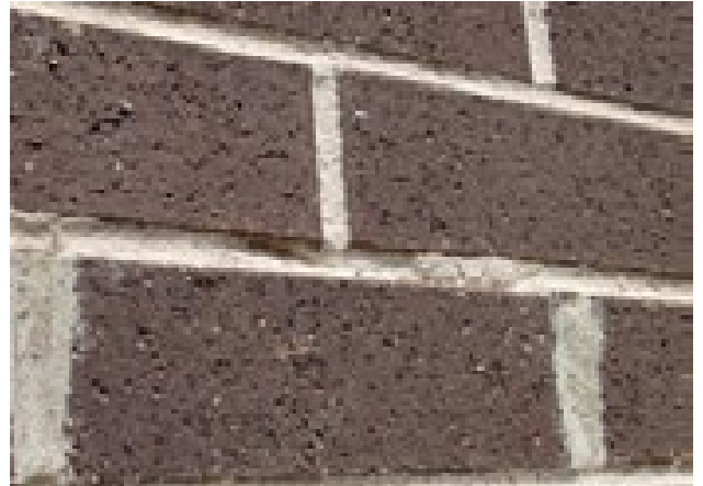
Figure 57 Damage caused by incorrect high pressure water jet cleaning
